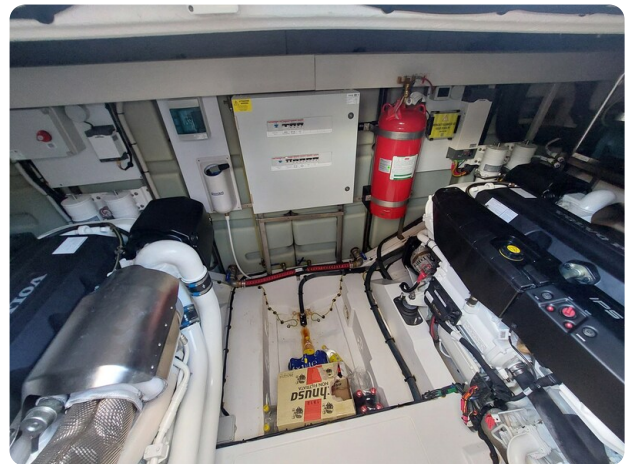
Azimut 53 Fly engine room
