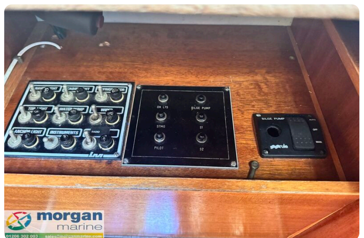
LM 27 Motor Sailer - switch panel
