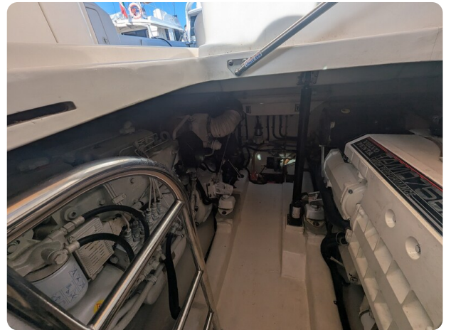
Riviera 4000 Offshore engine room
