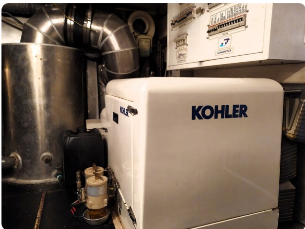
SANLORENZO SL 62 Generator
