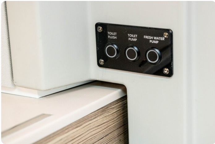
SAXDOR 270 GTO Electrical panel
