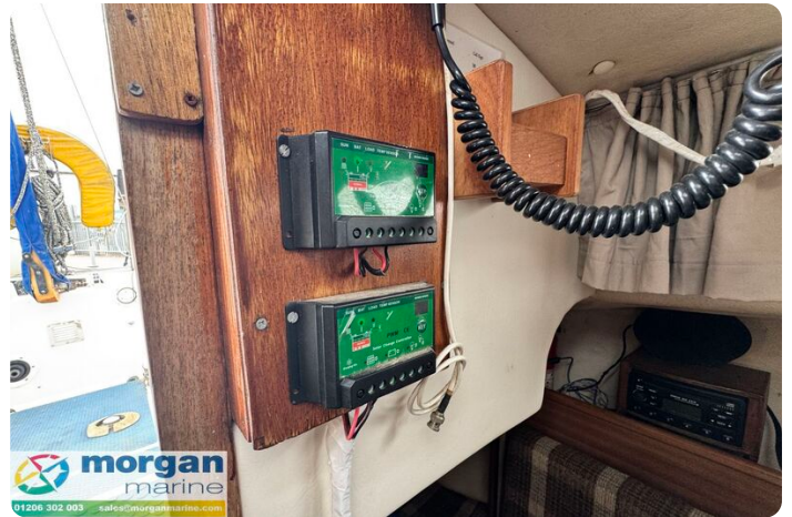
Westerly Griffon MK1 - solar charge
